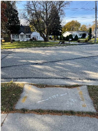
Non-Compliant Curb Ramps
